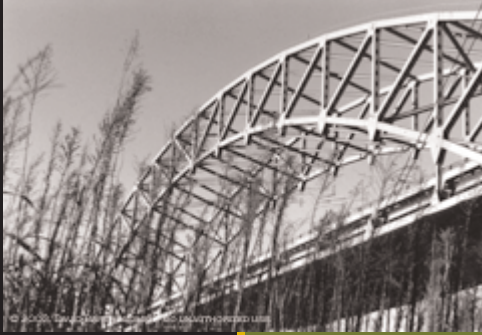
B28-27-C Bridge Over Amber Waves
